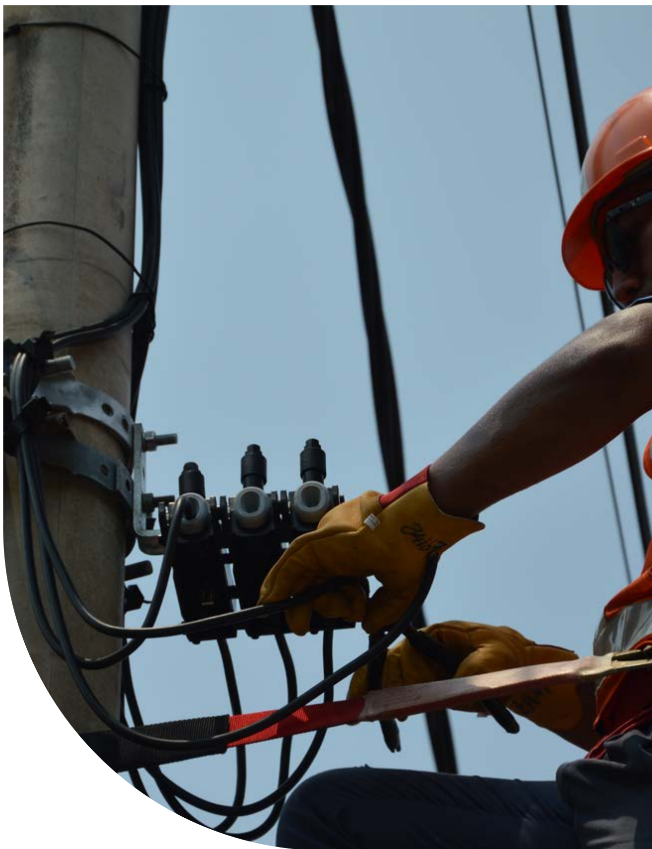
Fuse switch disconnecter MICHAUD installation - Tonga
