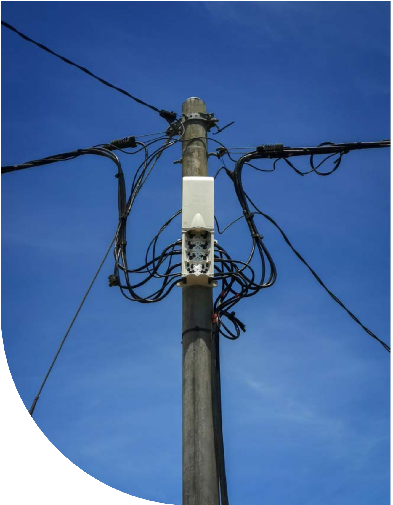
Aerial connexion box MICHAUD P429 - Malaysia
